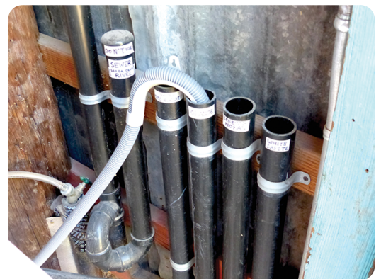
Brad Lancaster's washing machine grey water system. The outlet pipe from the washing machine can be moved to provide water to four different fruit trees. Photo by Andy Mason.
