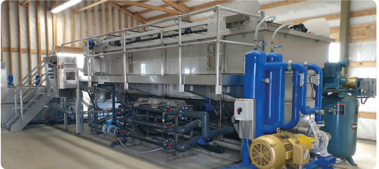
DVO dissolved air flotation nutrient recovery system.
